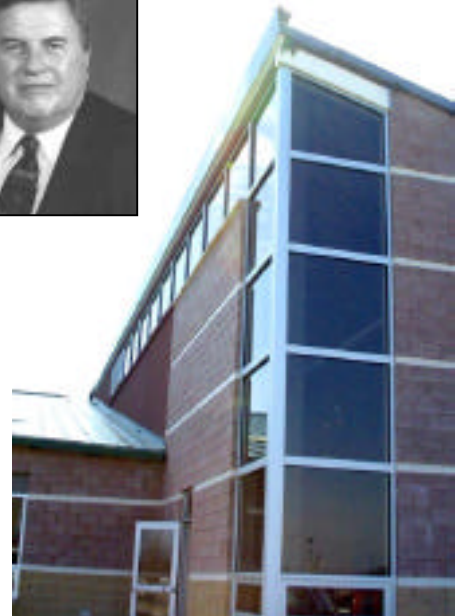
Above, a view of Robert Drummond Elementary, currently under construction, and a photo of the school's namesake.
